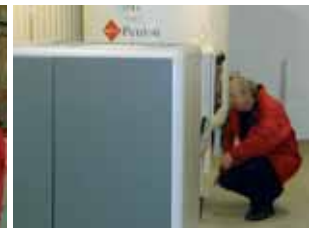
Medical Air Plant Servicing
